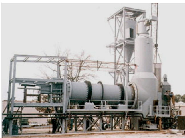
Picture 5 - Rotary Kiln Waste Incinerator Plant with Vertical Thermo-Reactor
